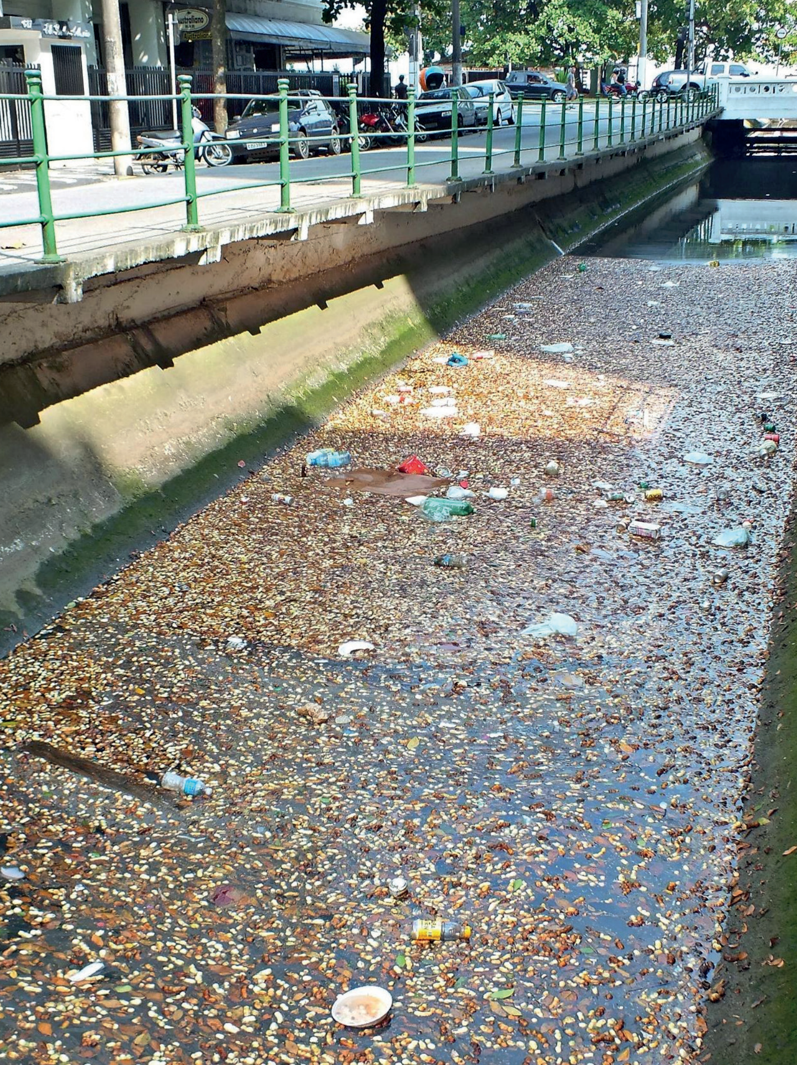
Figure 21. Solid waste found on Canal 4, between Boqueirão and Embaré neighborhoods. Photos: William R. Schepis.
