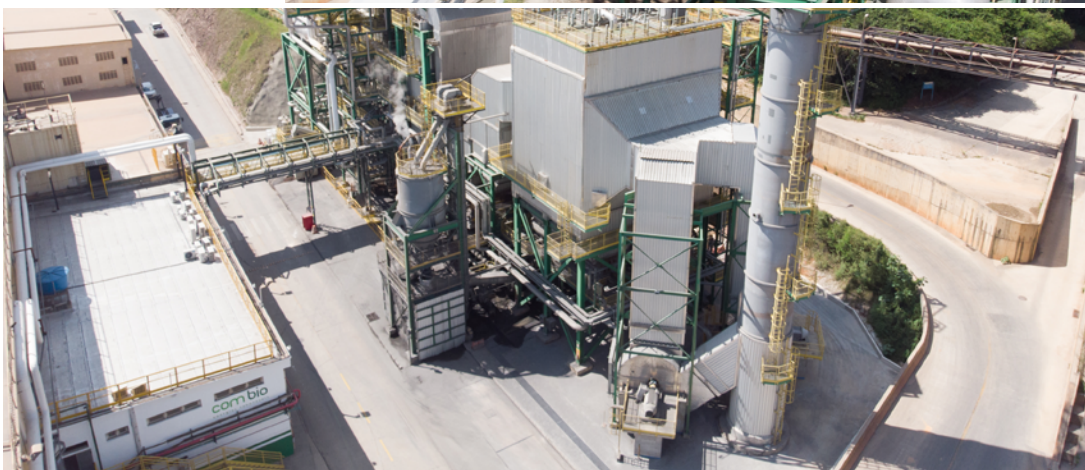
Biomass Boiler at the Alumina Refinery (municipality of Alumínio/SP).
