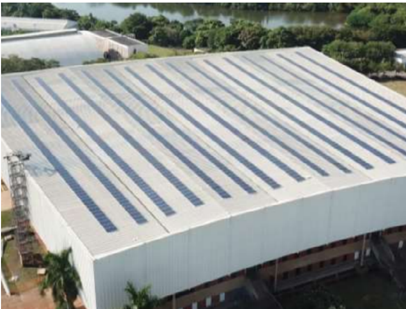
Photovoltaic System of the UNICAMP Gymnasium.
