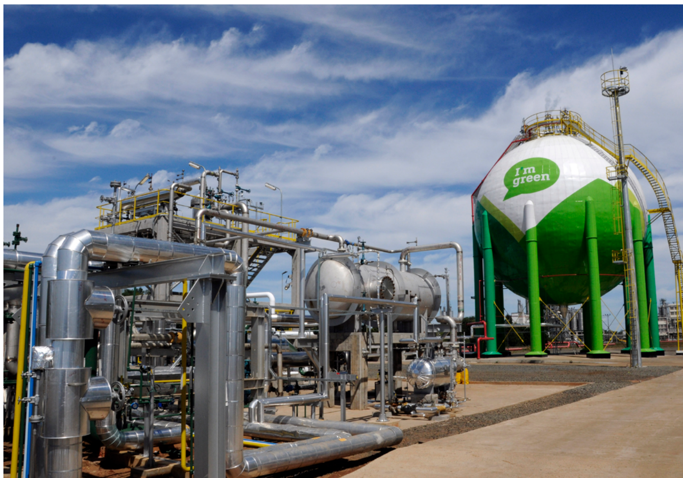
Green ethylene production at Triunfo, Rio Grande do Sul.
