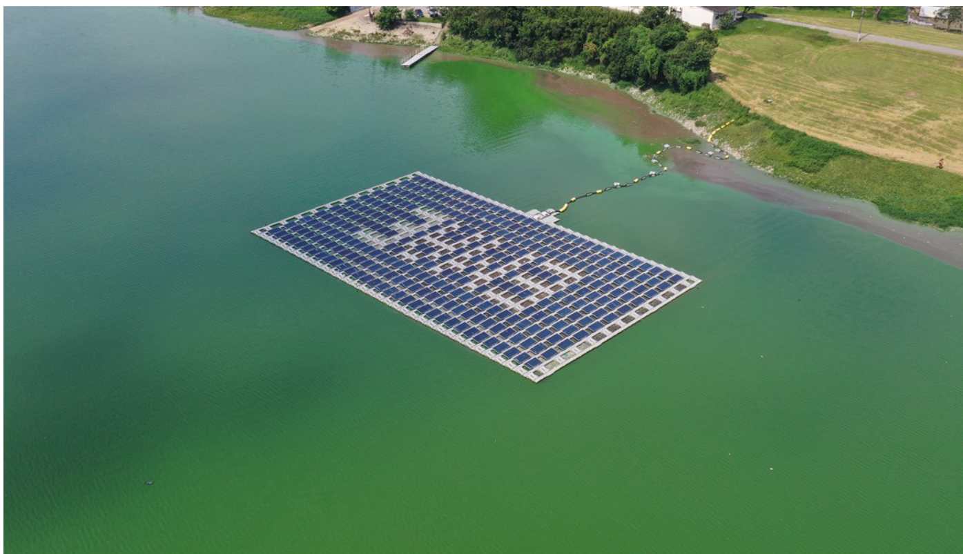
Floating solar power plant in Billings reservoir - aerial view.
