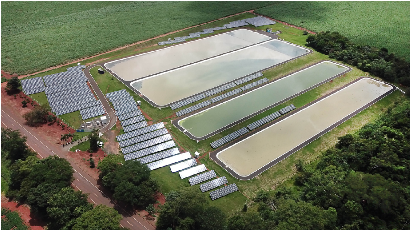
Photovoltaic plant for generating solar energy installed in the area of Sabesp's Sewage Treatment Plant in Orindiúva-SP.
