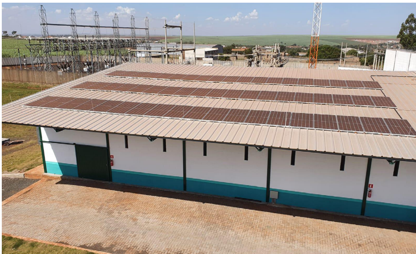
Empty Packaging Receiving Station in Guariba - SP with the installation of the photovoltaic solar power system on the roof.
